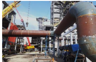
Biomass Power Plant
