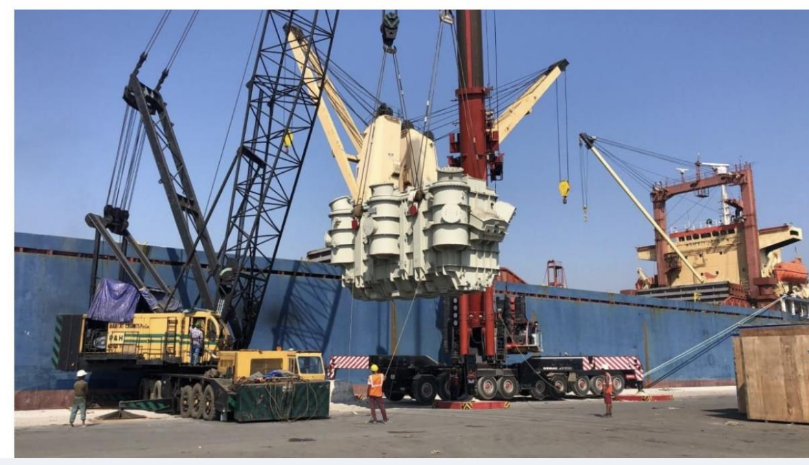
Transformers & Accessories moved for a Critical Substation project from India Factory to Tanzania Port by Total Move... www.theheavyliftgroup.com · 1 min read
